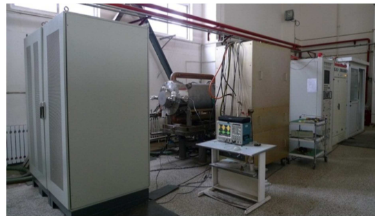
Fig. 7. View of the CSNS/RCS RF system prototypes.
